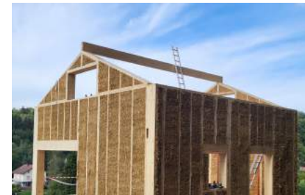
Ronchamp care facility, 37 tons of CO 2 secured.
